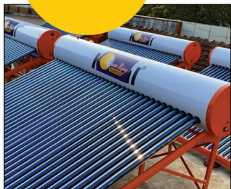
Solar Water Heater Colaco Hospital Mangalore
