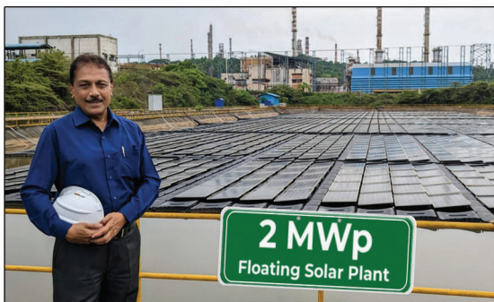
Floating Solar Power Plant
